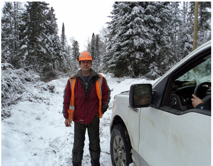
Figure 3.2: Mike Lesperance (Member of BNA) works along side the installers to install the hydro poles into Phase one (1) of housing.
